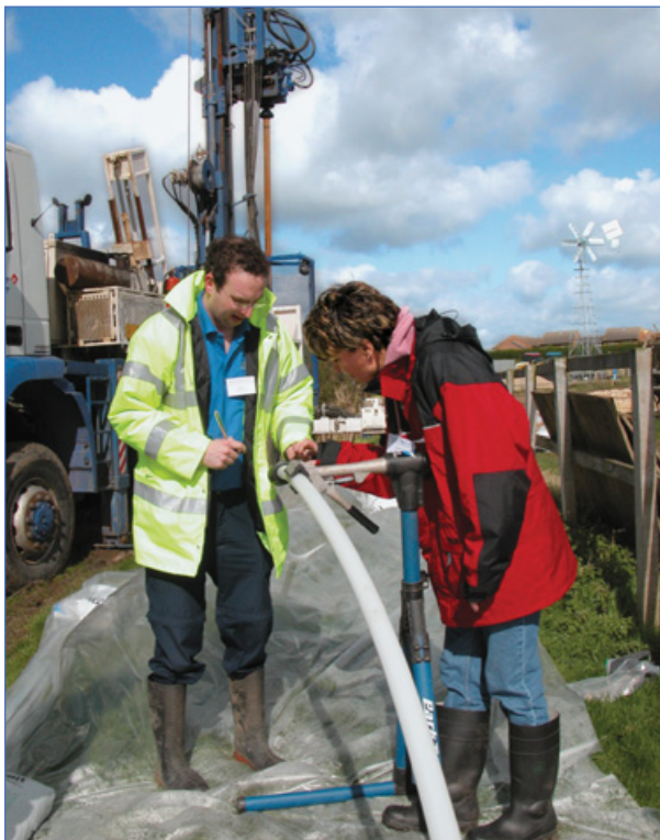
Construction of CMT ports in a 7-Channel System installed in Silsoe, England.
