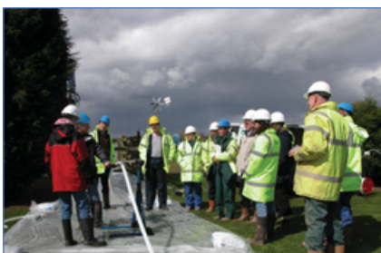
CMT Installation and training as part of a “Multilevel Course” given by the University of Cranfield at Silsoe, U.K., in conjunction with Wattera (UK), British Geological Survey & Norwest Holst.
